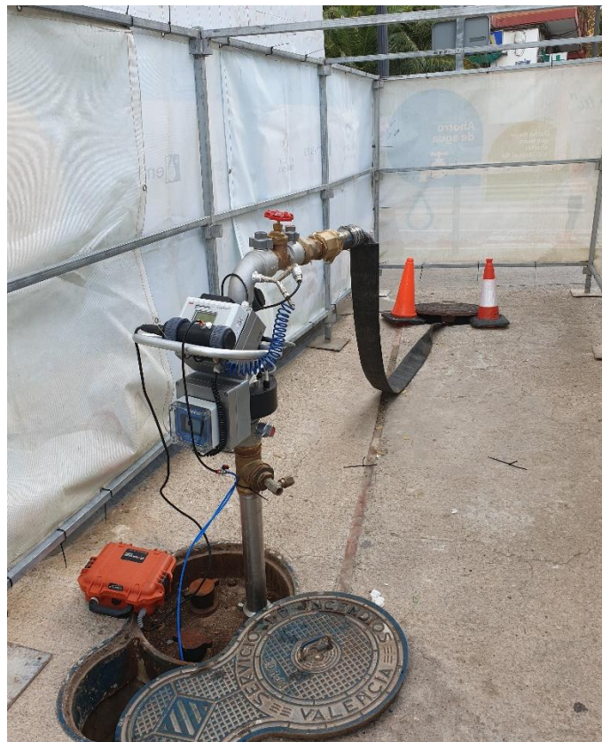
Figure 1 Flushing standpipe with flow, pressure and turbidity monitoring, 28 th November 2019
